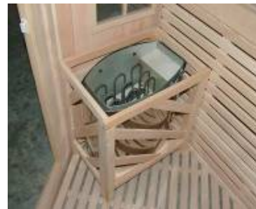
FIG-26 location of the stove
